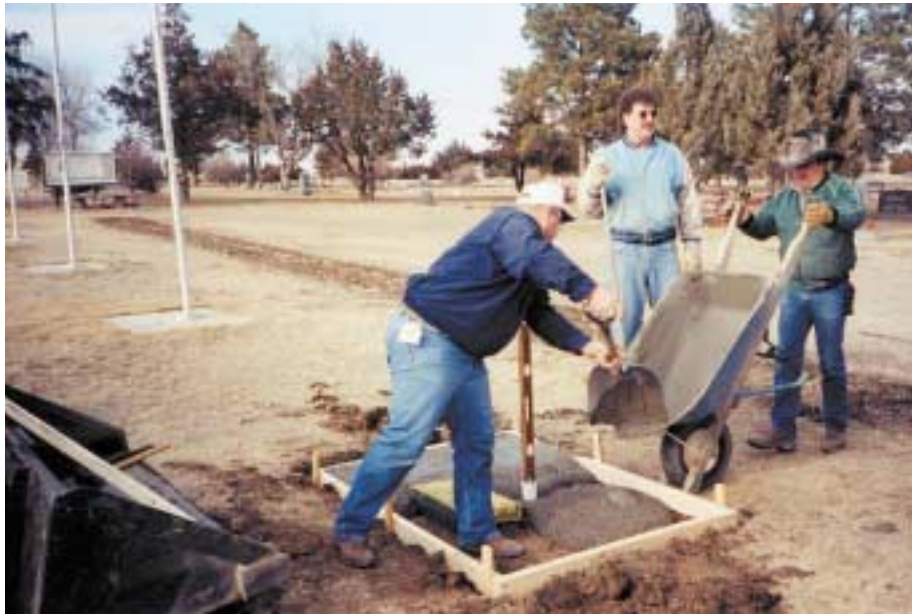
Lester Pearson pours a wheelbarrow full of cement as he, Don Haynes, and Mike Moses install a new flagpole, expanding the row of memorial flagpoles at the entrance of the Philip cemetery.
